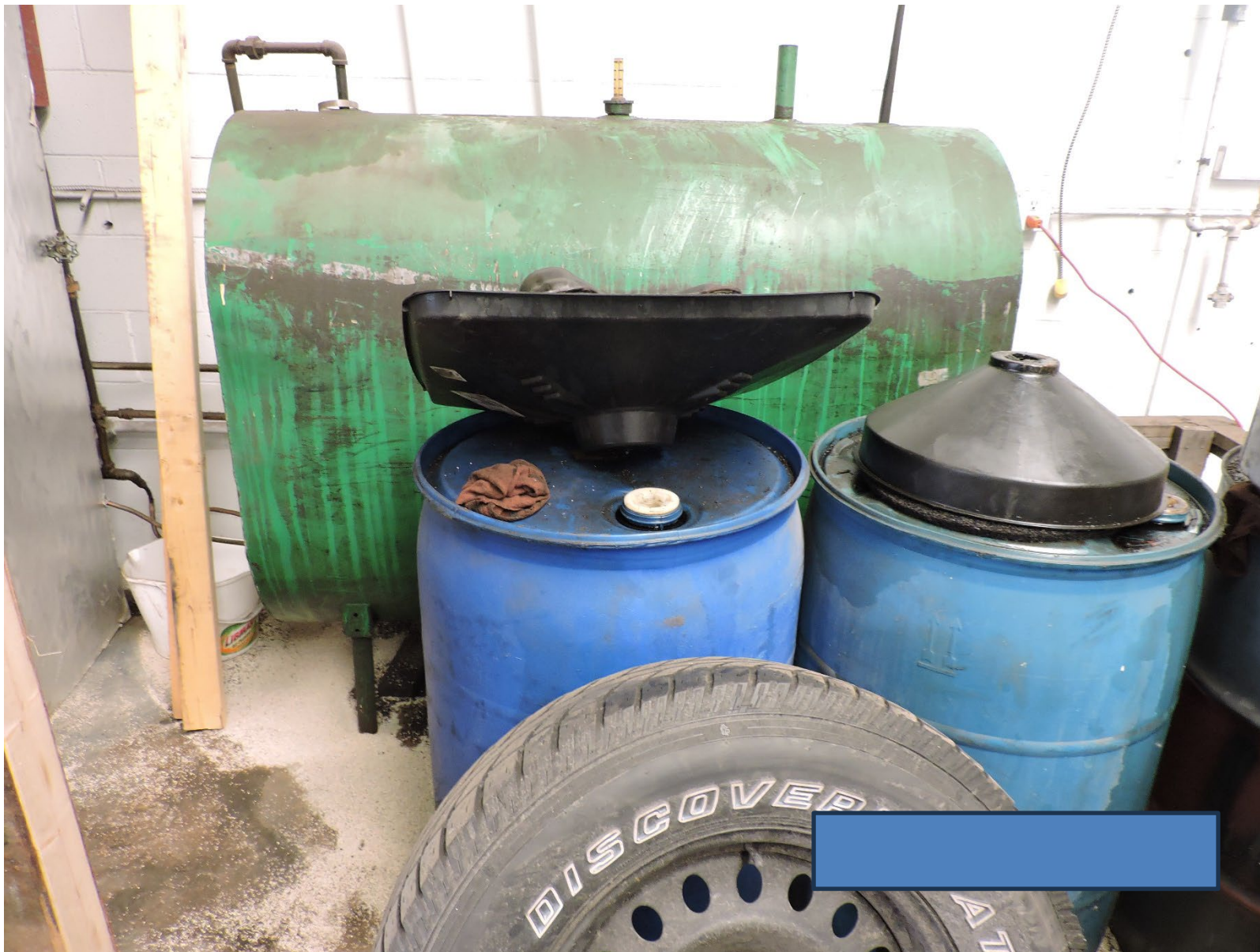
Unlabeled secondary containers.
