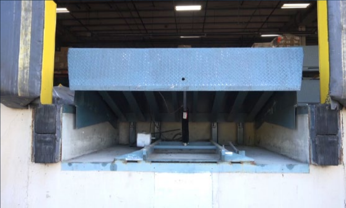
Confined Space: Crushing\collapse hazard
